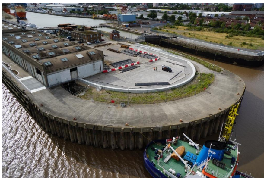
An aerial view of some of the new flood walls at Albert Dock
